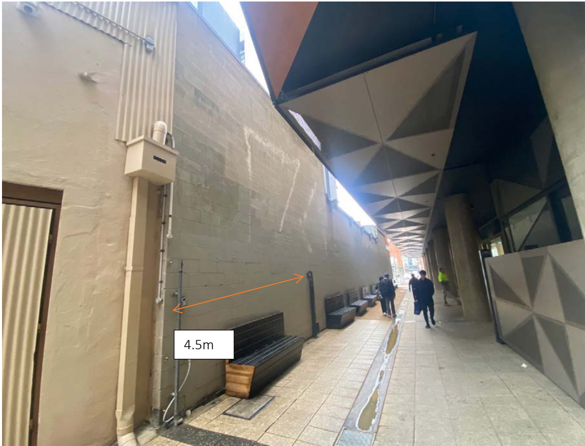
fig. 4 The wall from Playhouse Lane (artwork can be included in this section)
